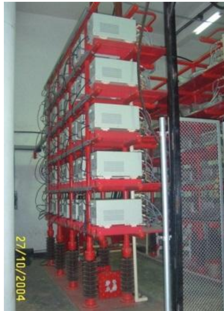
HV generated by Switched Power Modules
